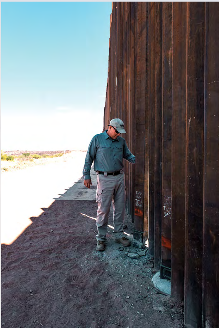
The author inspects a breach in the wall.
